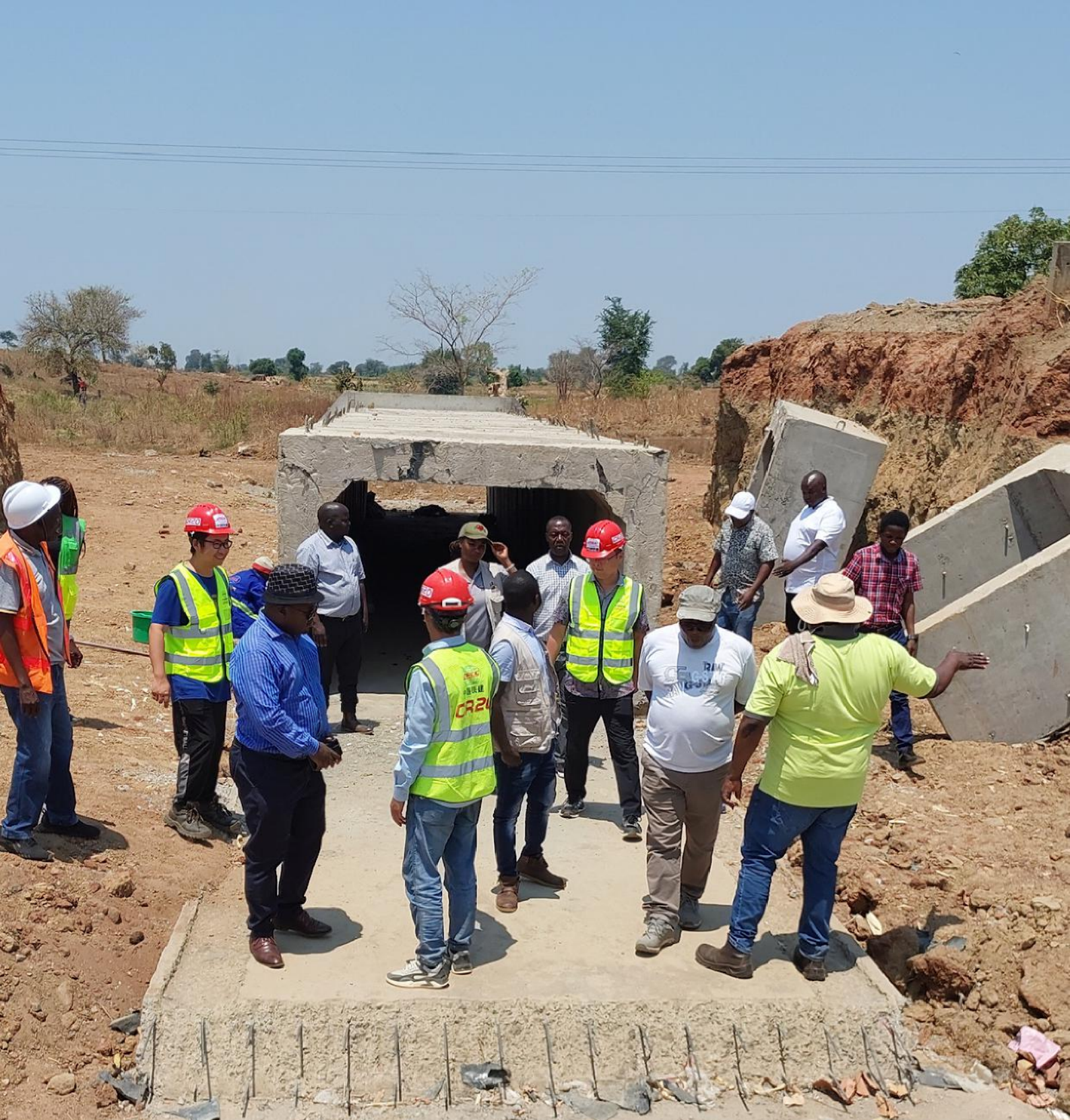
A site meeting with contractor CR20 and Consultants working on the Salima Nkhotakota M5 Road
